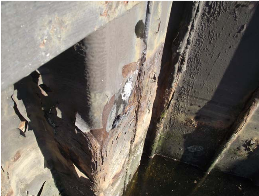
Typical tidal zone metal loss
