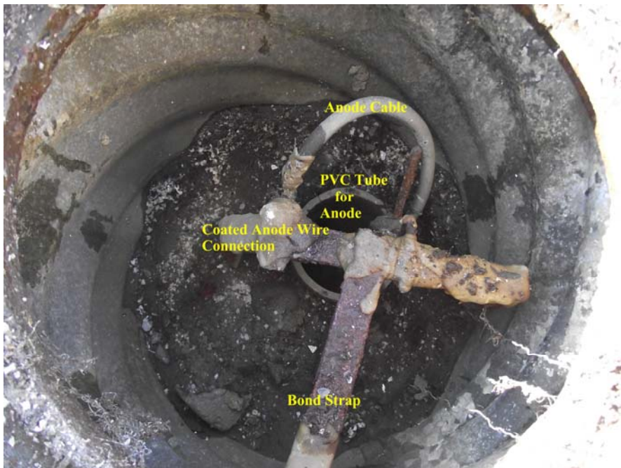
Typical CP Station
