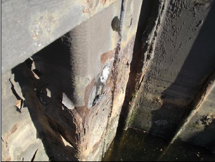
Typical severe corrosion and layering in tidal zone
