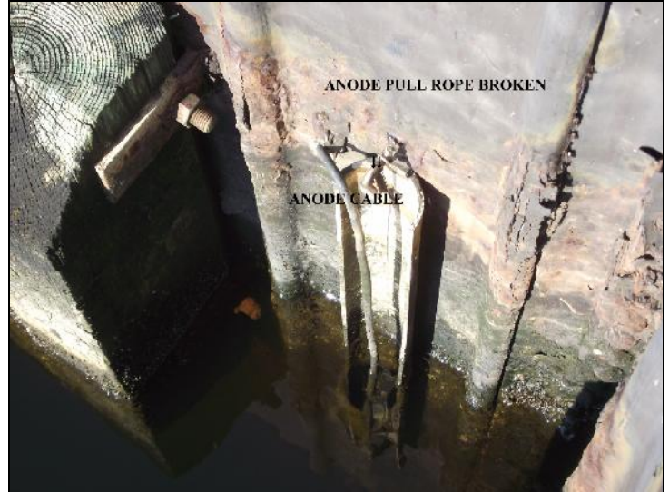
Typical water side anode installation
