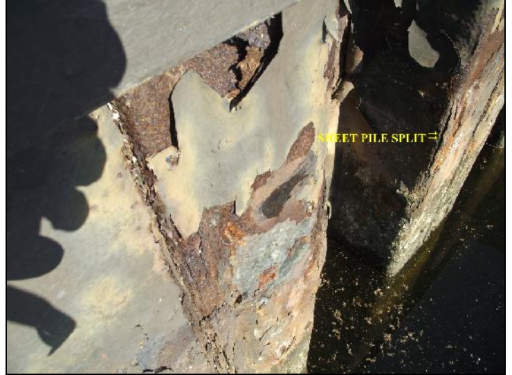
Deep layer corrosion and splitting on corner bend of sheet
