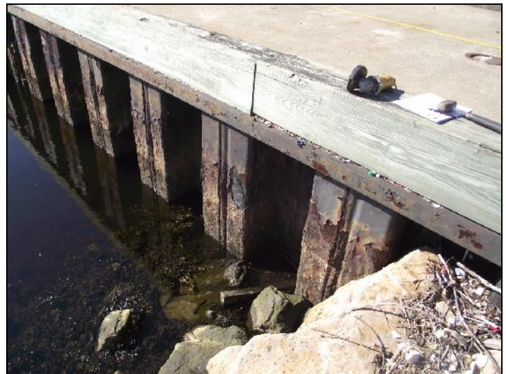
East end of sheeting, tidal zone corrosion is apparent
